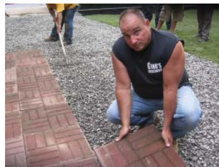
The King of Dirt being filmed installing a walkway in an up coming episode.
